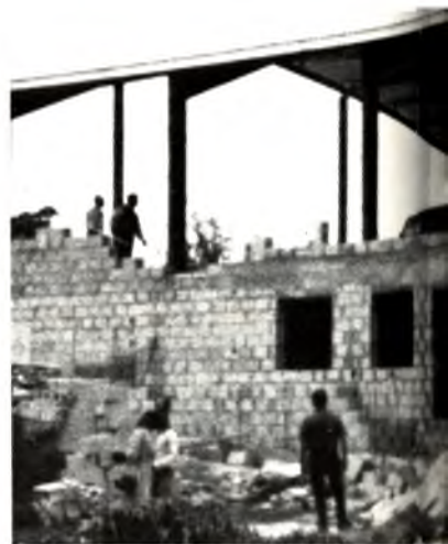
The Collymore Rock Church (above) in Barbados being rebuilt by the Work and Witness team from Pasadena, Calif., First Church.
