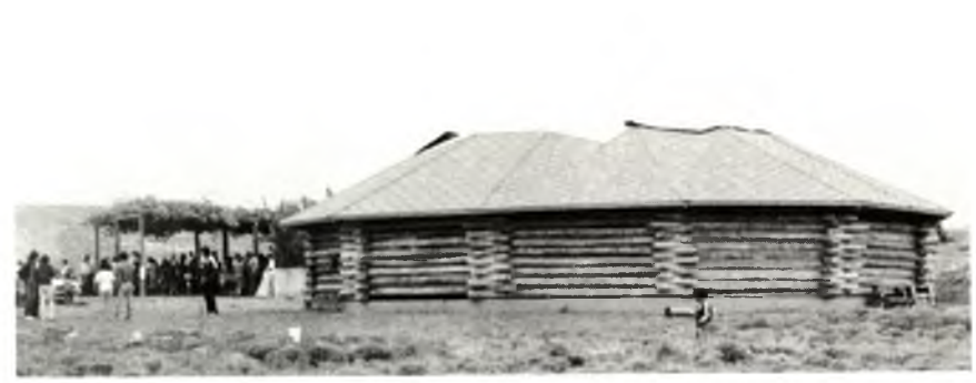
The exterior of the hogan-style log structure, shown partially completed, is the home for the new Nazlini, Ariz., Navajo Indian church.
