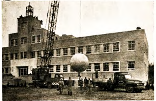
EIGHT-FOOT GLOBE being raised to the top of the new international headquarters building in Kansas City, Missouri. Globe was made for the Nazarene headquarters building by Mr. Dallas Meade, artist, of Tulsa, Oklahoma.
